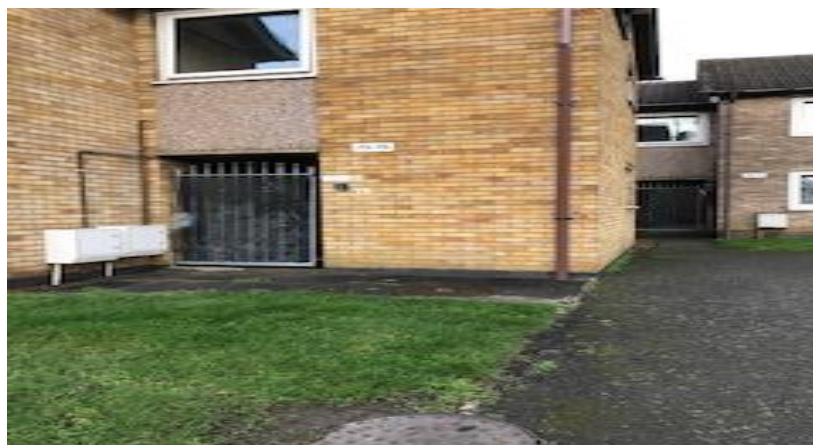
Dupont Gardens – The gates need upgrading. There is a need to upgrade these gates, they are old and rusty and to add intercom for additional security for tenants and residents living in the block
